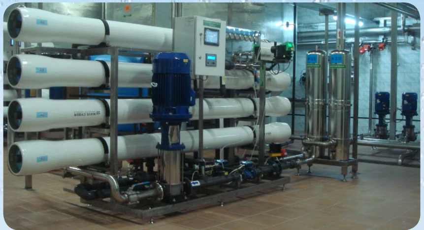
Water purification systems of Ecofil LLC used in food industry
